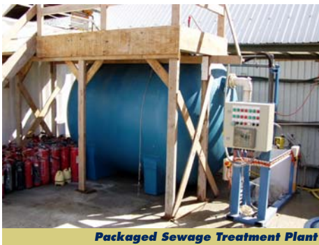
Packaged Sewage Treatment Plant
