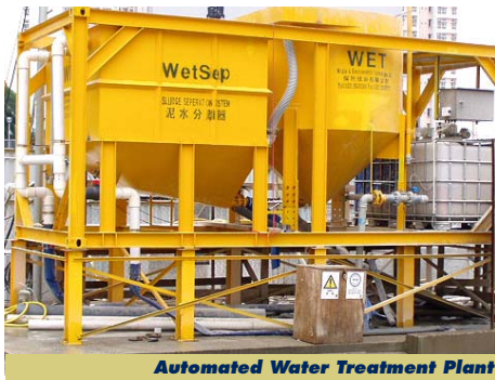
Automated Water Treatment Plant
