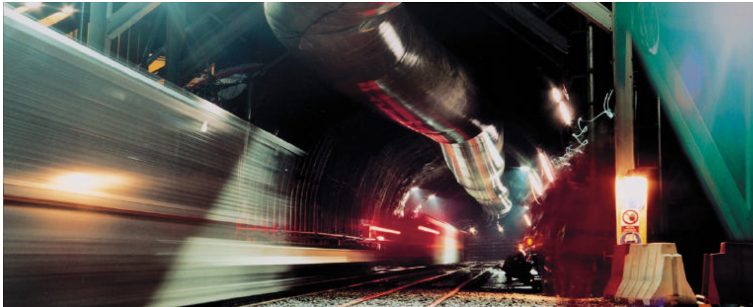
St. Gotthard Base Tunnel – the world's longest rail tunnel. Together with four partners, HOCHTIEF is building approx. 30 kilometers of the tunnel's 57 kilometer total length. Due for completion in 2014.
